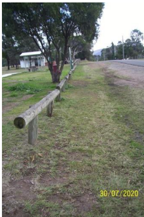
Pot holes along outside parking area need maintenance
